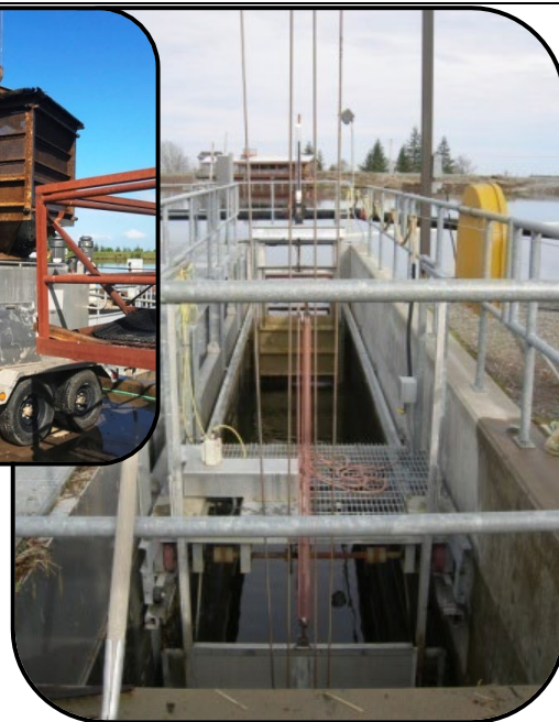
Electron Hydro fish collection facility (trap), and water-to-water fish transfer into hauling trailer.
