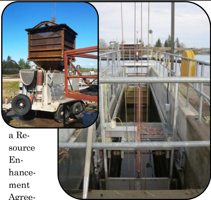
Electron Hydro fish collection facility (trap), and water-to-water fish transfer into hauling trailer.
